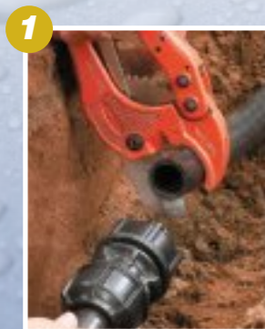
1 Cut the pipe square. There is no need to chamfer or lubricate the pipe.
